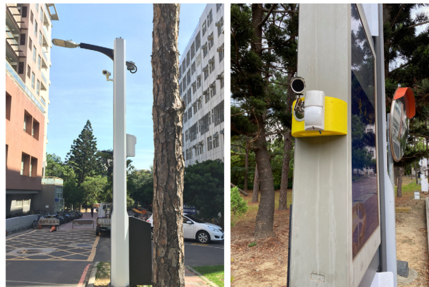
Fig. 9. Our testbed at NTHU campus, Taiwan: a smart street lamp (left) and a motion sensor (right).
